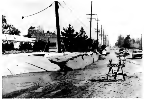
Photo 20. Foothill Nursing Home on Foothill Boulevard, Los Angeles. Sidewalk has been raised 3 feet by faulting with respect to the street. The Ledger (La Cañada Valley) photo.
